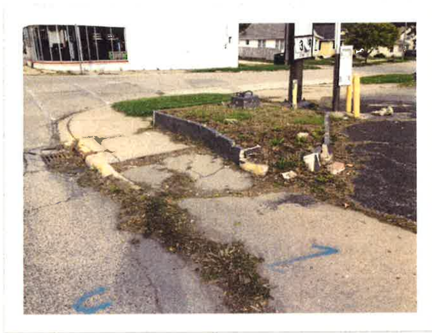
Looking west approaching Warren Avenue. At photo showing the need for full replacement of sidewalks and curbs.
