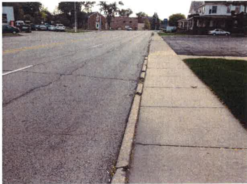
Looking East near Belvidere Funeral Home. Note the lack of any water carrying capacity in the curb that has been overlaid to the top. Also note broken curb head.
