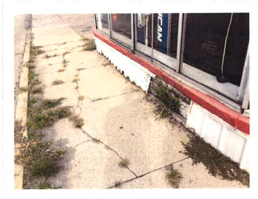
A photo at F and F Tire Service showing more sidewalk and curb repair needs. Here the business owner needs to also coordinate some work on his building.
