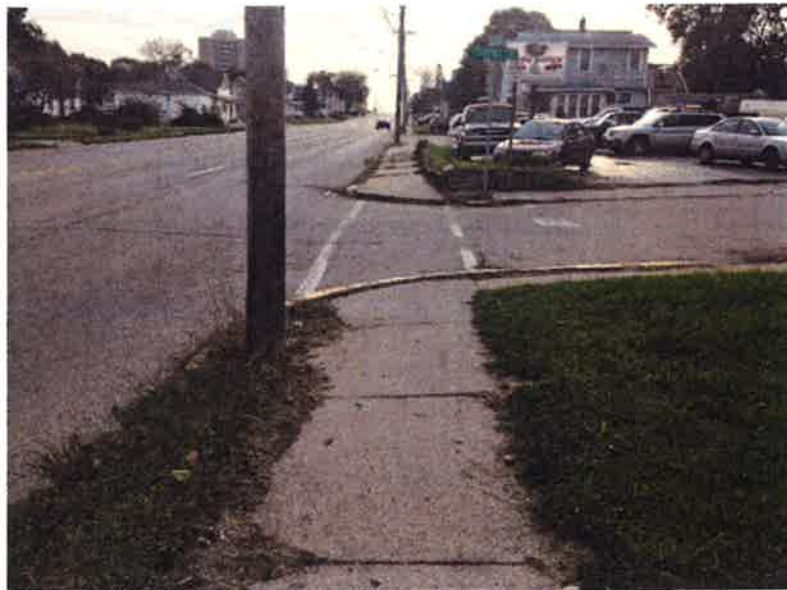
Looking East @ Florence Court. Note the lack of ADA ramps and the power poles encroaching on the sidewalk
