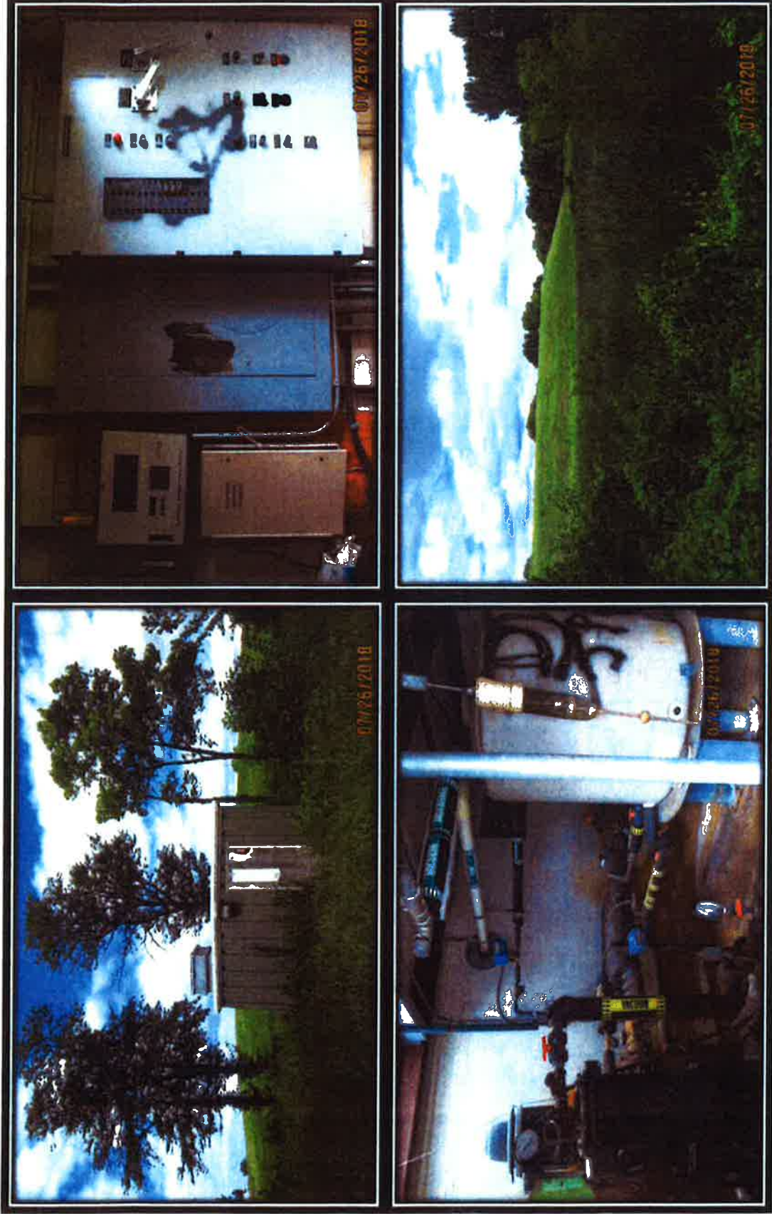
Figure 4. Site Photographs. Pump house with vacuums and equipment for pumping extraction wells (top left); control panel for equipment operation (top right); Vacuums and extraction equipment, single suction pumping system with force main connection to City sanitary sewer system (bottom left); View of landfill, looking southeast from detention area (bottom right).
